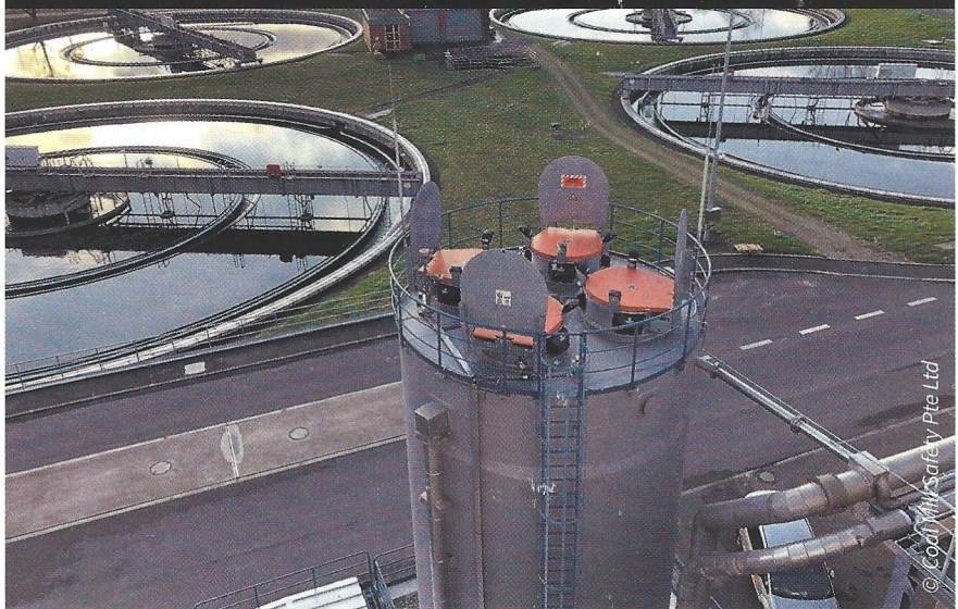
Figure 3: example of a correctly-protected dried sewage sludge silo with explosion pressure shock resistance and accessible self-reclosing explosion vents
